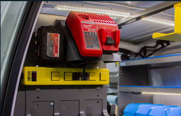
BATTERY CHARGING STATION
